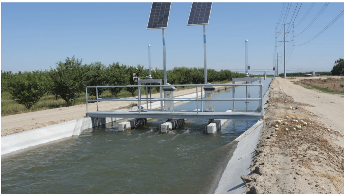
The solar-powered automated flume gates communicate among themselves as well as the 70 or so automated side gates to regulate canal flows and save water.
